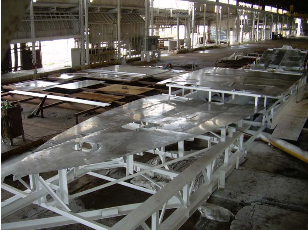
A ship's hull begins to take shape in the Industrial Canal shipyard United States Marine is leasing from Trinity Yachts. United States Marine has been in Gulfport since its eastern New Orleans shipyard was destroyed in Hurricane Katrina, but it is using the New Orleans facility to fulfill a defense contract.
